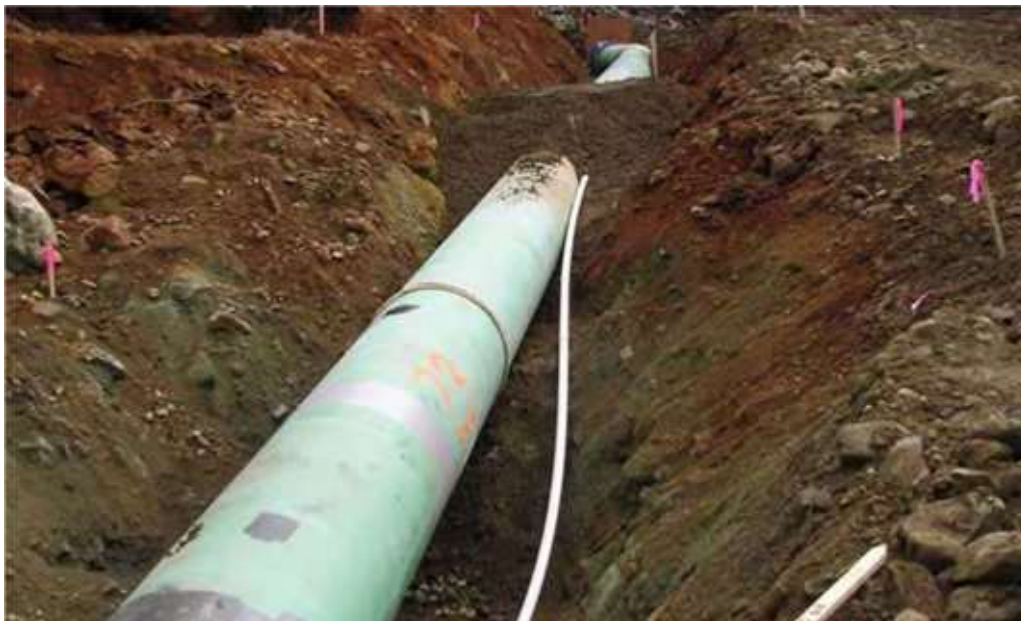
Figure 3-14: Photo of buried steel piping with Victaulic couplings
